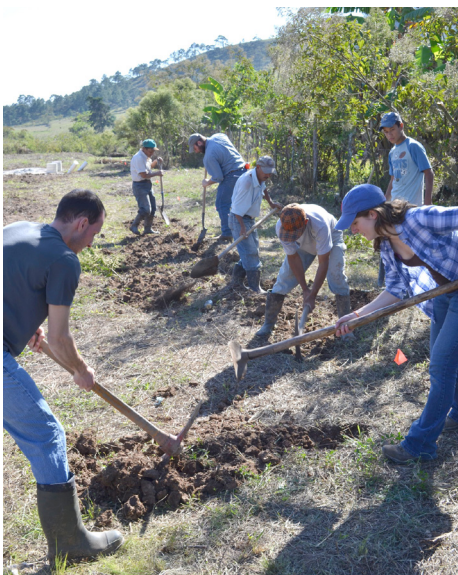
Engineers Without Borders' student chapter at the University of Maine has been concentrating on improving sewage treatment and disposal in Dulce Vivir, Honduras.
