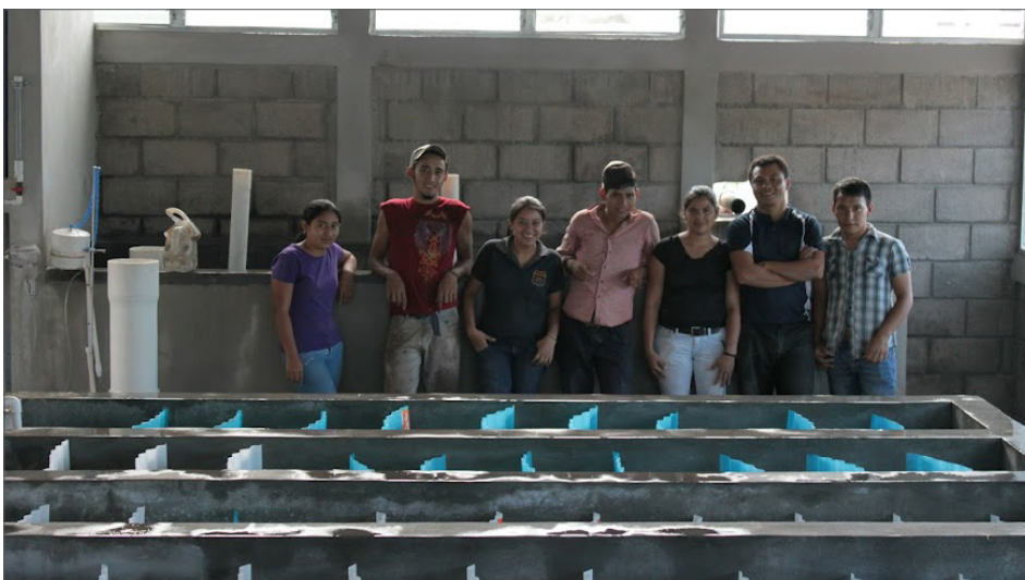
AguaClara’s Atima, Honduras plant will be completed this year, bringing safe, clean water to the community.
